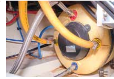
The hot water cylinder showing the lower tube feeding cold water into the tank (blue collar). The hot water output is at the top (red collar) and there are two yellow tubes that take hot water from the engine into and out of the cylinder (yellow collars).
