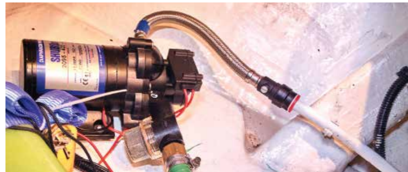
The accumulator should be as near to the water pump as possible. Fortunately, there was room for a 5lt accumulator adjacent to the pump with ready access to the pipework
