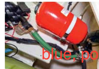
The accumulator in place near to the water pump. The flexible hose connecting the accumulator to the new T-piece in the fresh water system is shown in the top right of the picture
