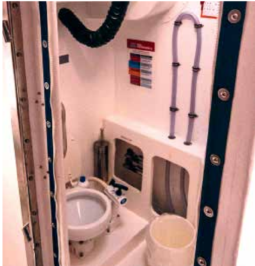
Keeping the workings accessible in the heads means an easier fix if things go wrong
