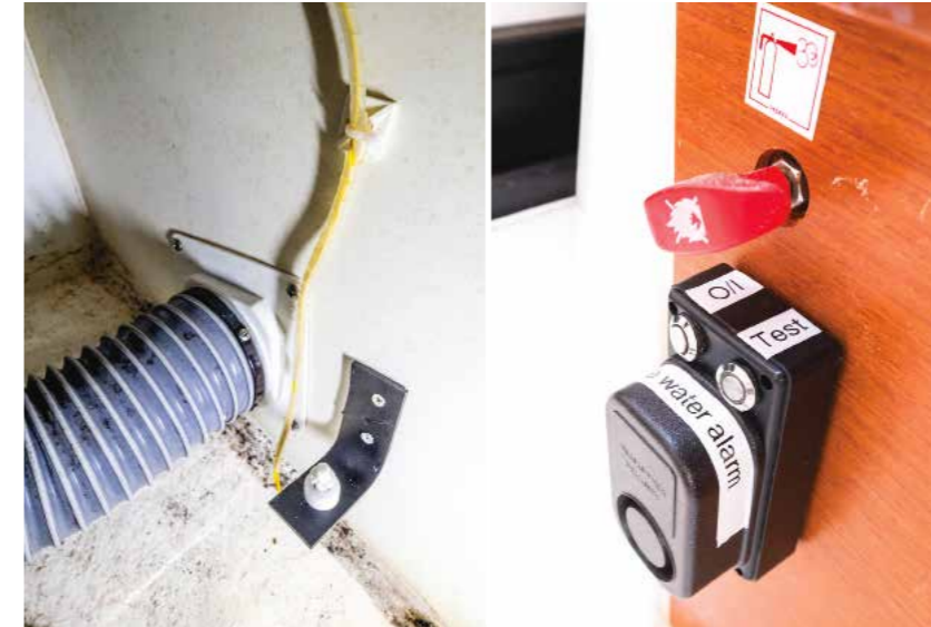
ABOVE LEFT The float switch in position in the bilge. The bracket is made from scrap acrylic, drilled for the screws and the float switch. Make sure you know which way up the switch has to go to work properly. ABOVE RIGHT The fitted bilge alarm siren. Note the on/off and test switches fitted into the box and the siren mounted on top of it
